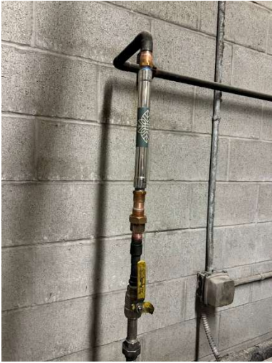
Shaft on Boiler Makeup Line
