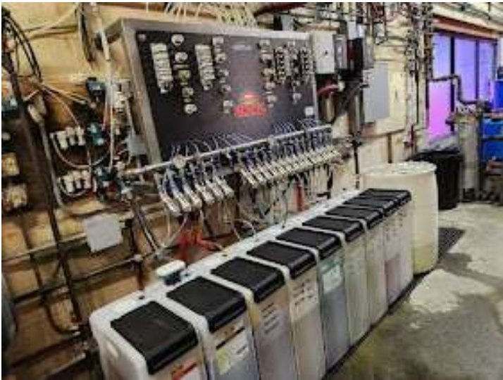
Shaft on car wash chemical dispensing system
